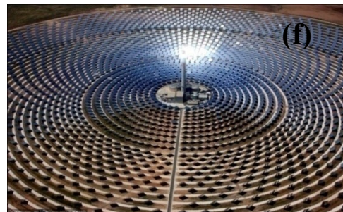
Solar power tower
