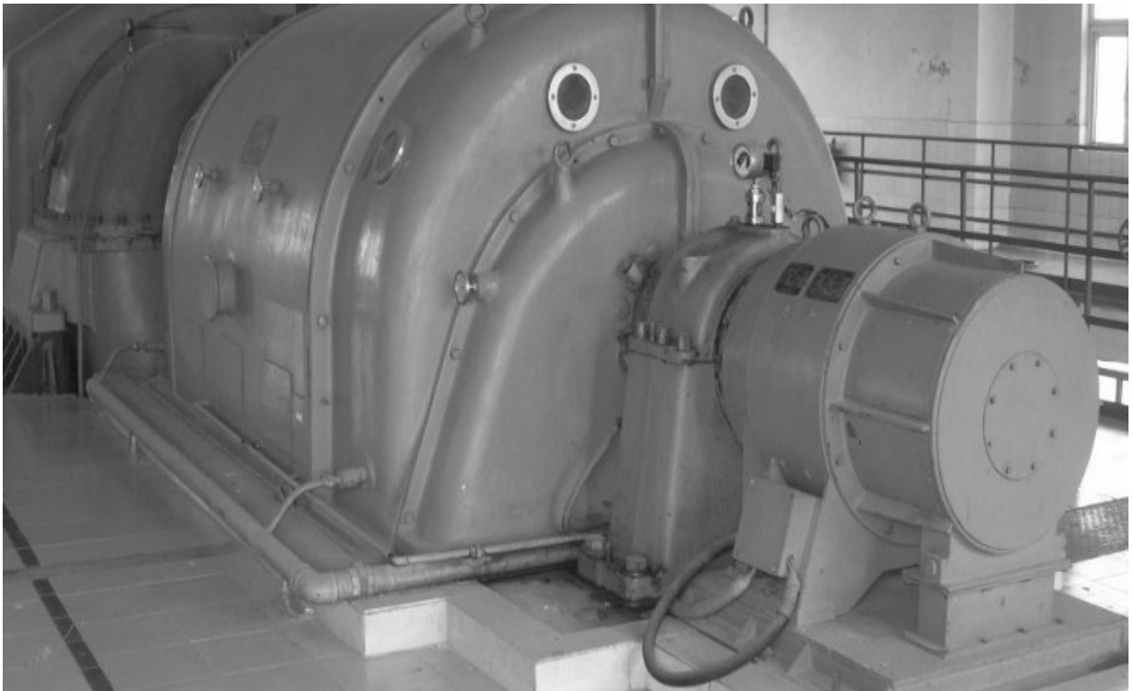
Figure 3.4 Turbine of G.H.T.P
