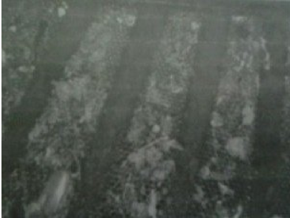
Figure 3.11 Blocked Condenser Tubes
