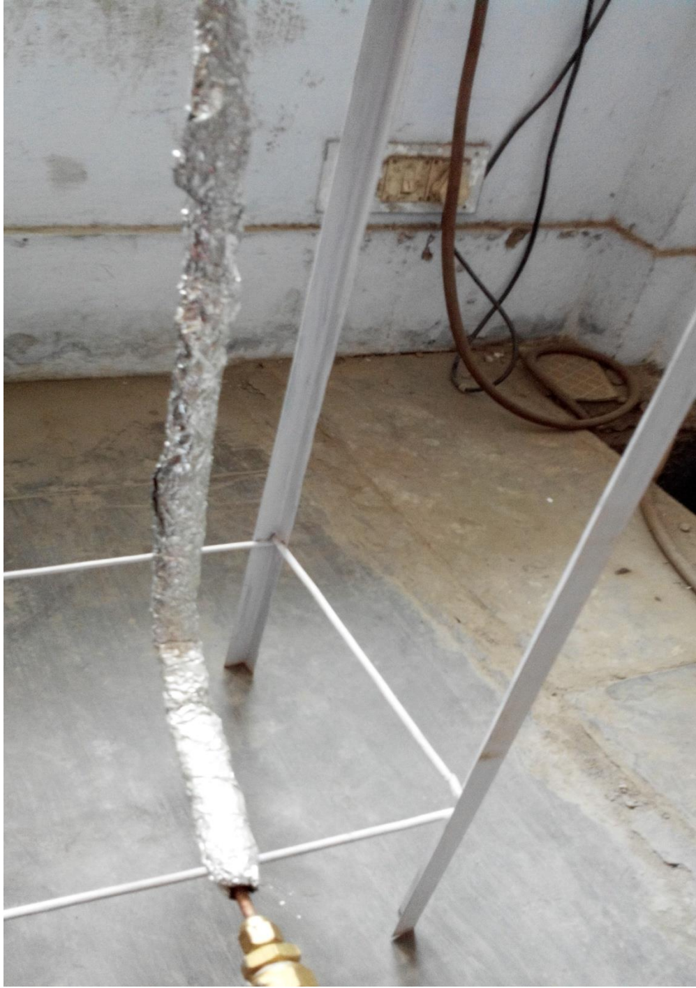
Insulated part of pipe.
