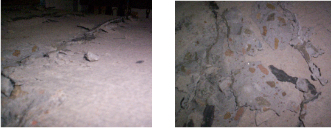
Fig 4.14 Photo showing failed concrete in compression at the top surface.
