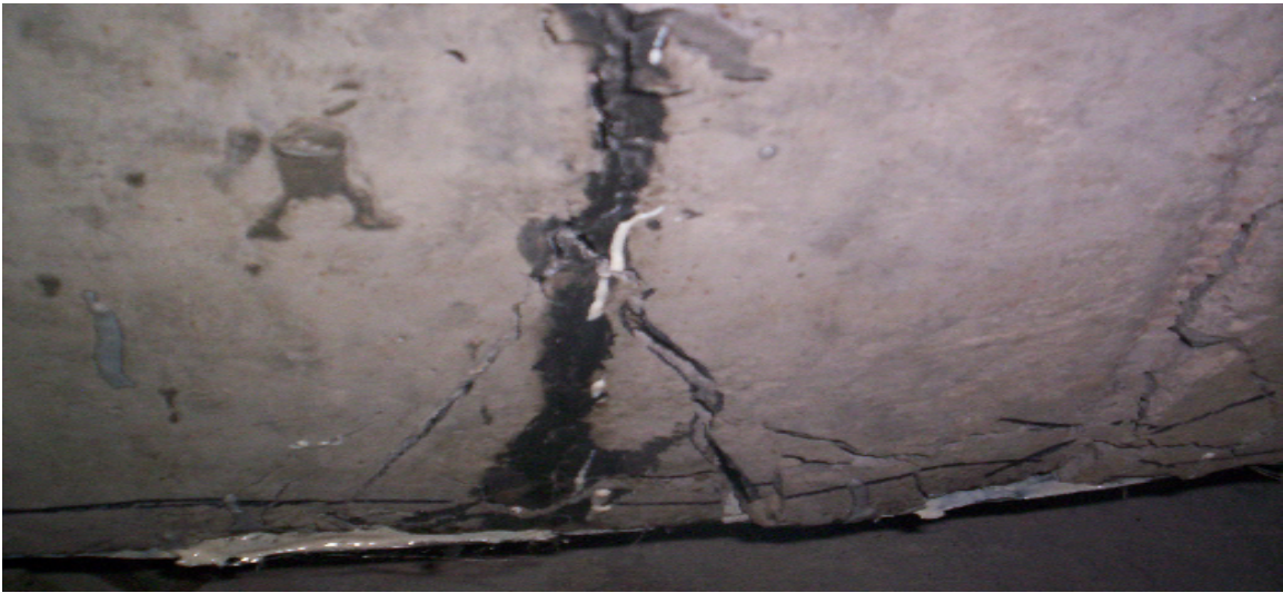
Fig 4.15 Photo showing crushed concrete just above the laminate; widen cracks & new cracks at bottom.
