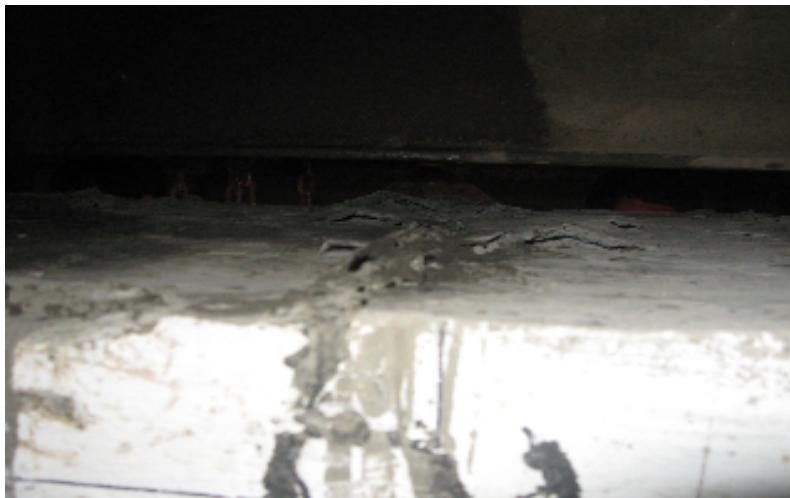
Fig 4.8 Photo showing concrete failure in compression at top surface
