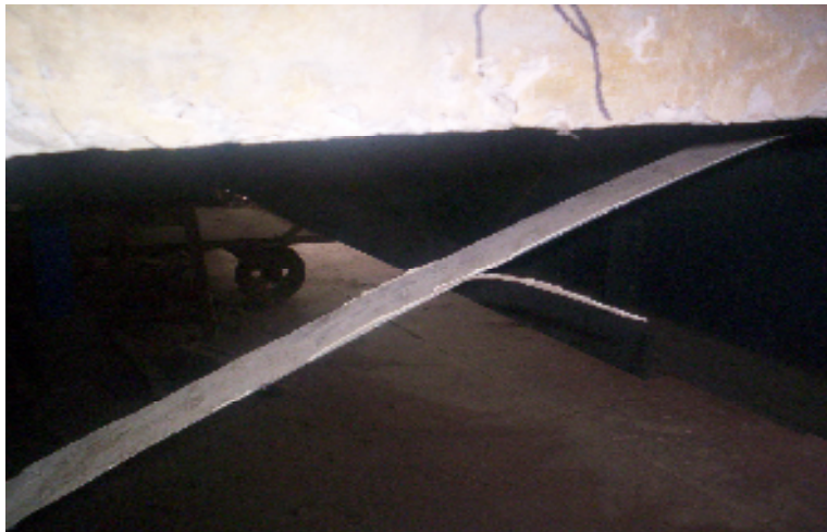
Fig 4.4 Beam with two laminates failed by interfacial debonding.
