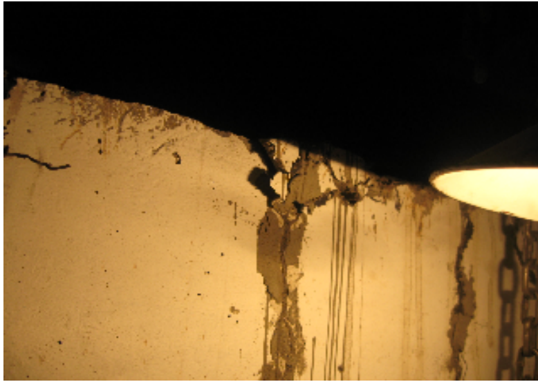
Fig 4.7 Photo showing starting of spalling at the top surface.
