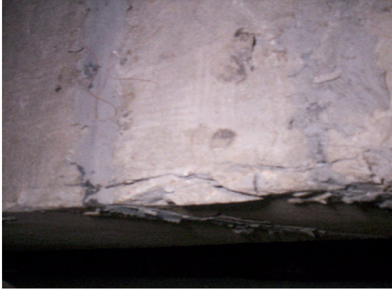
Fig 4.3 Starting of spalling at the bottom surface
