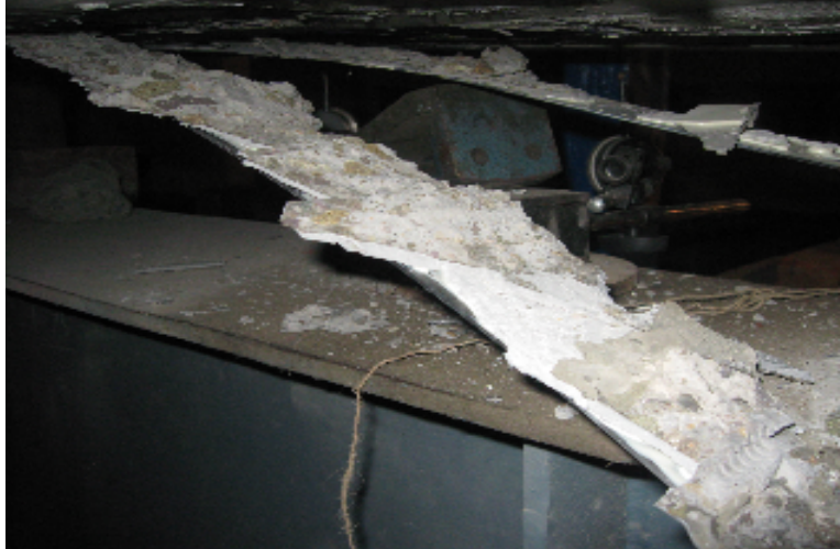
Fig 4.9 Photo showing failure of the beam by partial peeling off & debonding of laminates
